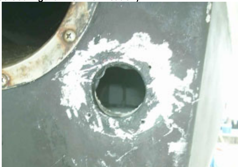
Figure 1- Old Thru-Hull Location
