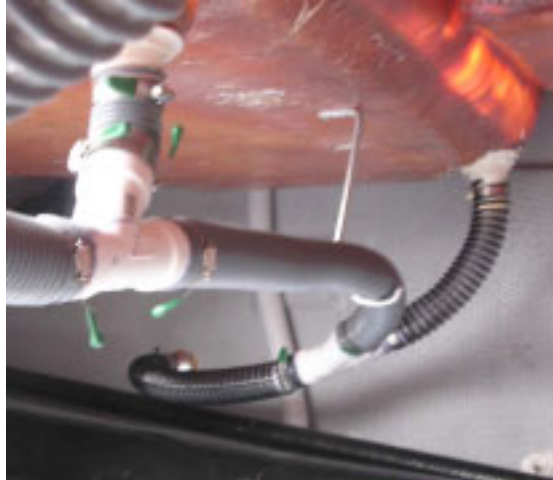
Figure 2- New Hose and Thru-Hull Configuration
